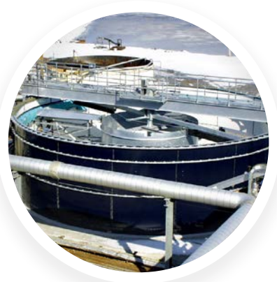
Municipal Wastewater Clarifier / Sludge / Storage / Mixing
