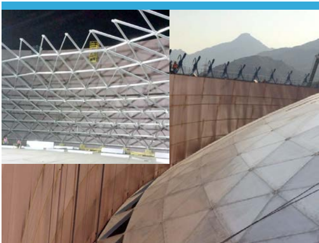
» National Water Company Makkah, Saudi Arabia – 361' Diameter
